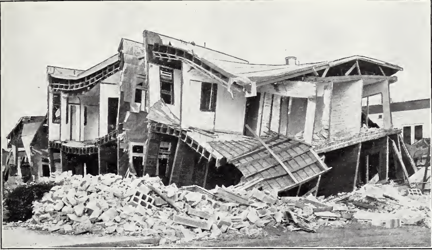
J. COLLAPSE DUE TO LACK OF TIE BETWEEN WALLS AND FRAME, THIELE BUILDING (CEMENT BLOCK), PALO ALTO.
